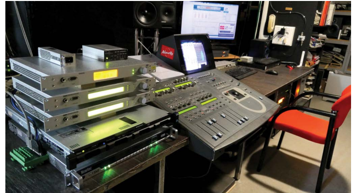
Alouette's engineering lab where devices are tested and evaluated.
